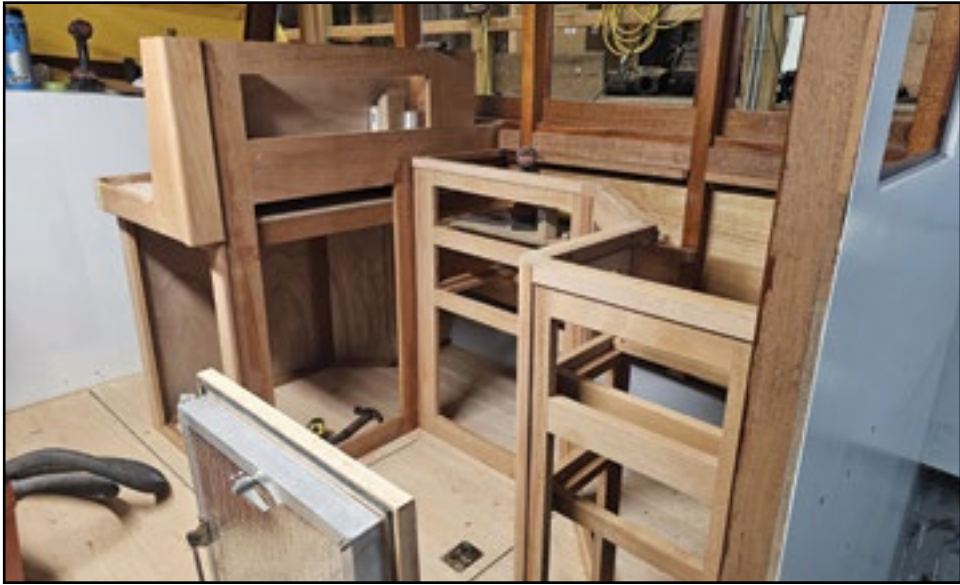
This a view into the main salon showing the roughed in interior of the former SUSAN JANE, which is being converted into a pleasure cruiser at John's Bay Boat in South Bristol.
