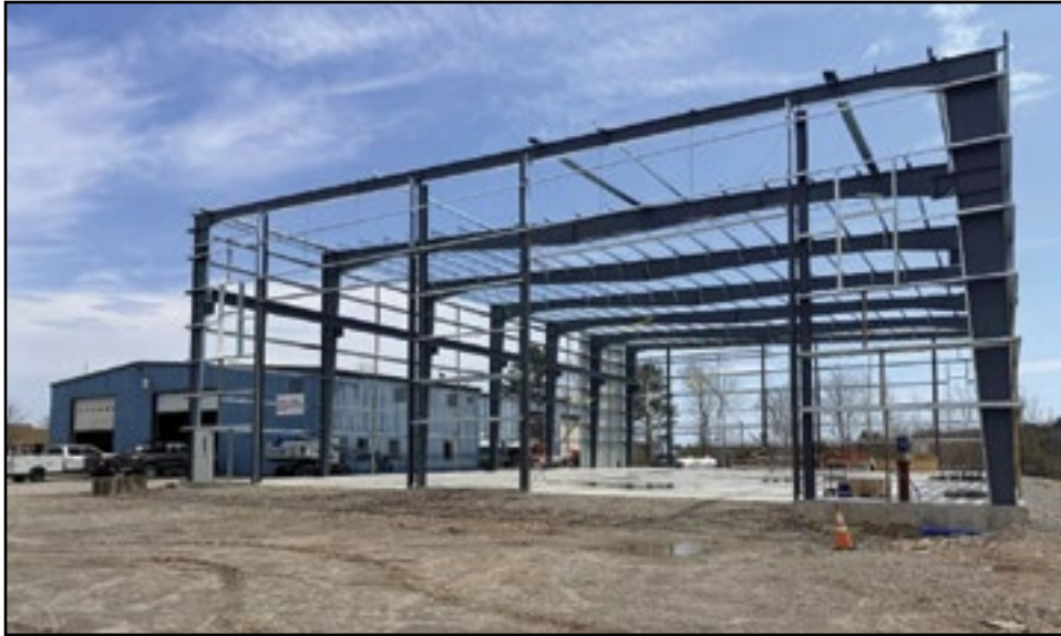
This is the new facility being erected by Lyman-Morse in Rockland. This is right next to the fabrication shop.
